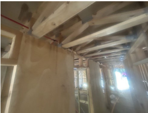
Internal braced walls were missing shear blocks, contrary to AS 4440 – 2004 Clause 2.2.3.
