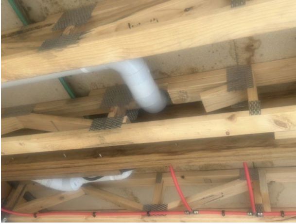
Floor truss webs were cut to allow for plumbing services.
