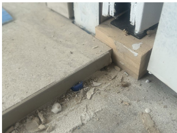
Floor level openings where waterstops and perimeter flashings are incorrectly installed.
