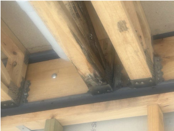
Various floor trusses had significant signs of degradation due to exposure.
