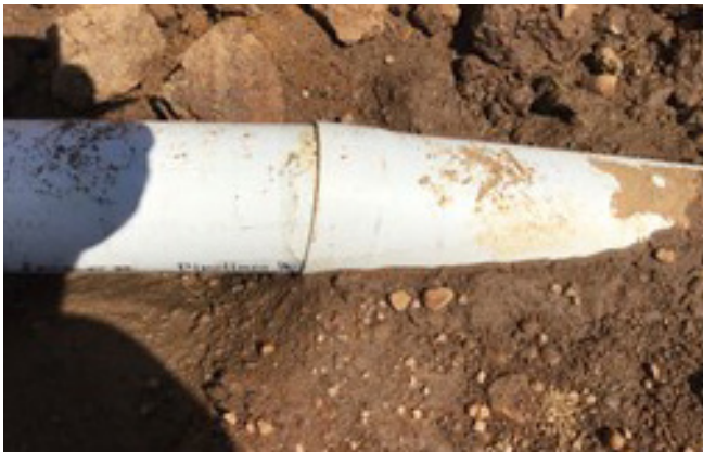
Fitting used for the installation of the stormwater drain has not been fully inserted.
