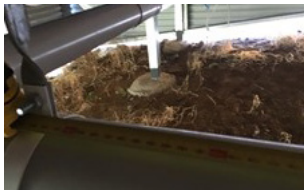
Suspended sewer without the appropriate support.
