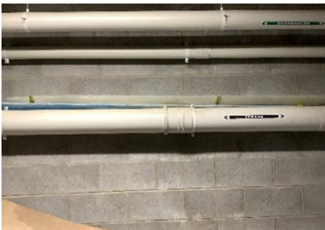
Expansion joints used without fixed supports
