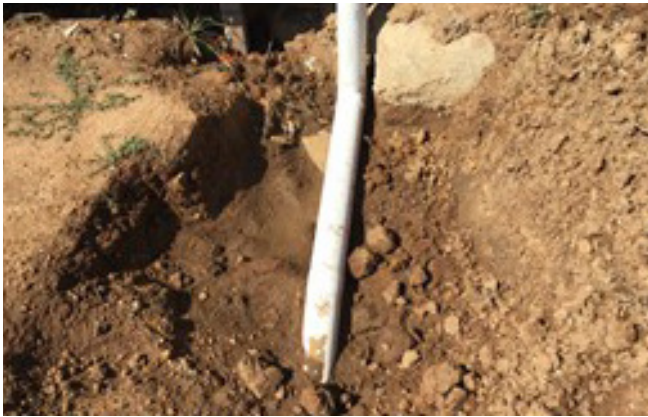
Below ground stormwater drain without the appropriate bedding/side support material
