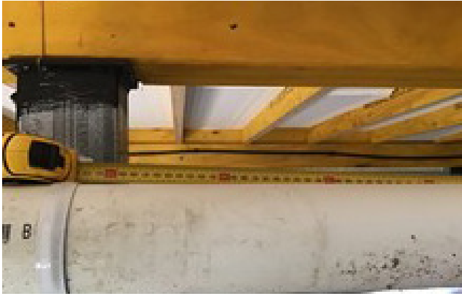
Above ground PVC stormwater without support at appropriate intervals.
