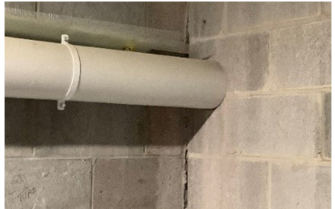
Drain through brick wall without the 25mm clearance
