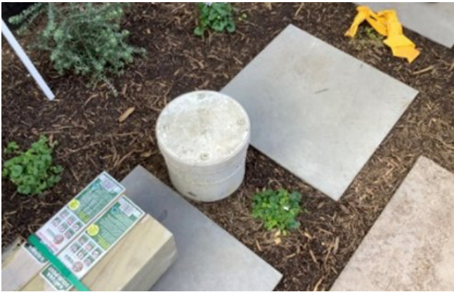
Unprotected plumbing fixtures
