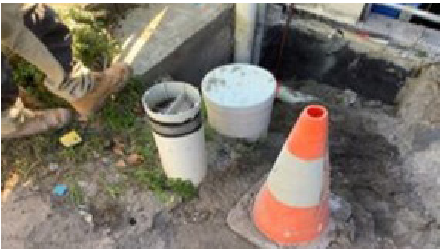
Non-compliant positioning of Reflux Valve
