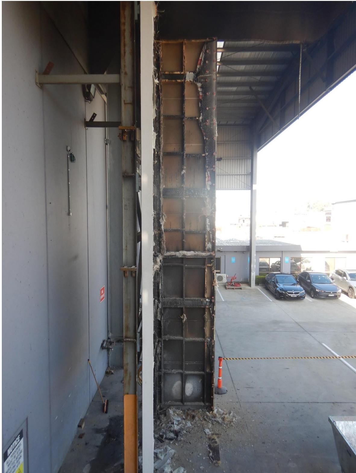
Figure 48 The post-test external wall system with all render removed – wing wall
