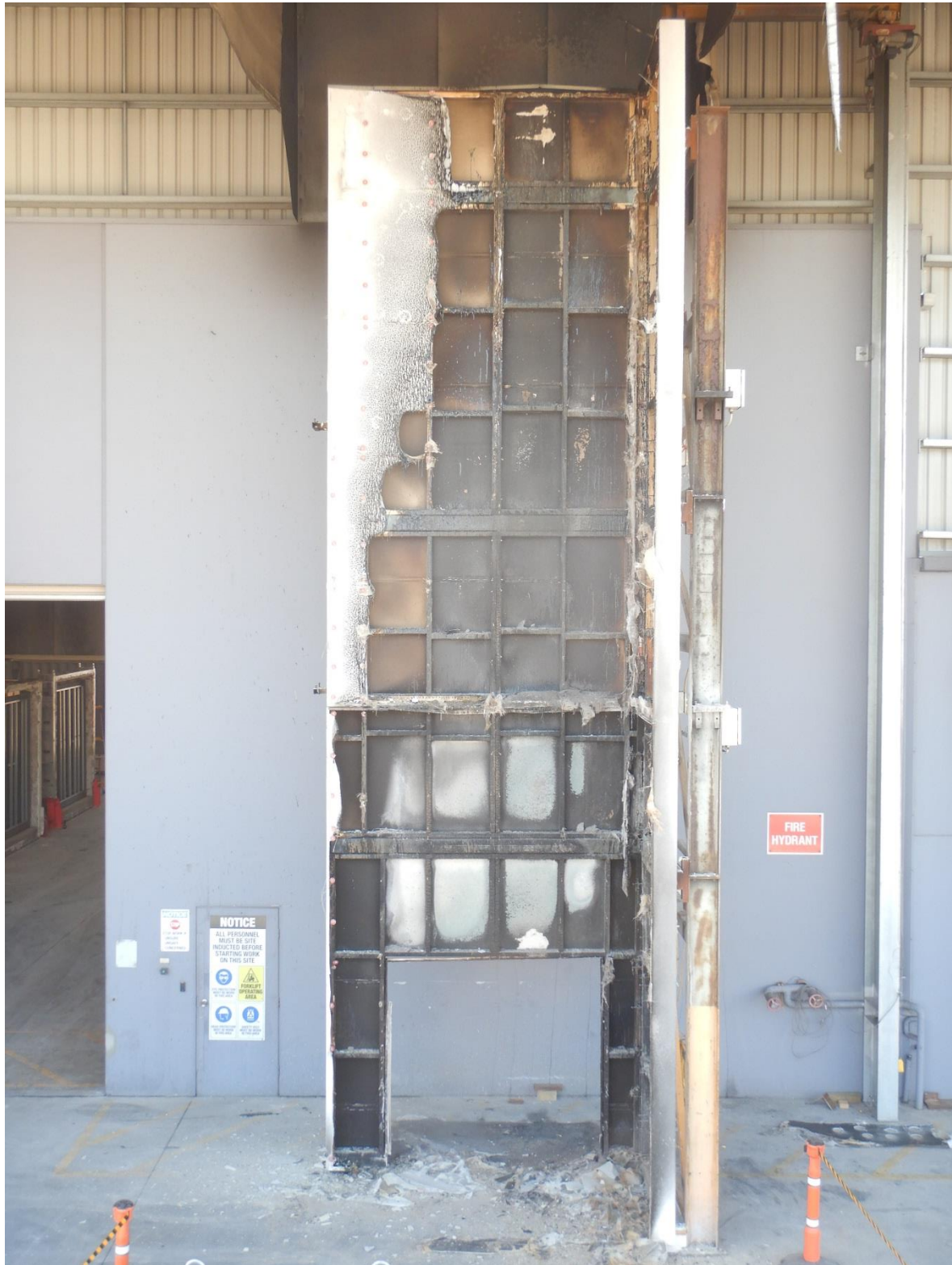
Figure 47 The post-test external wall system with all render removed – main wall
