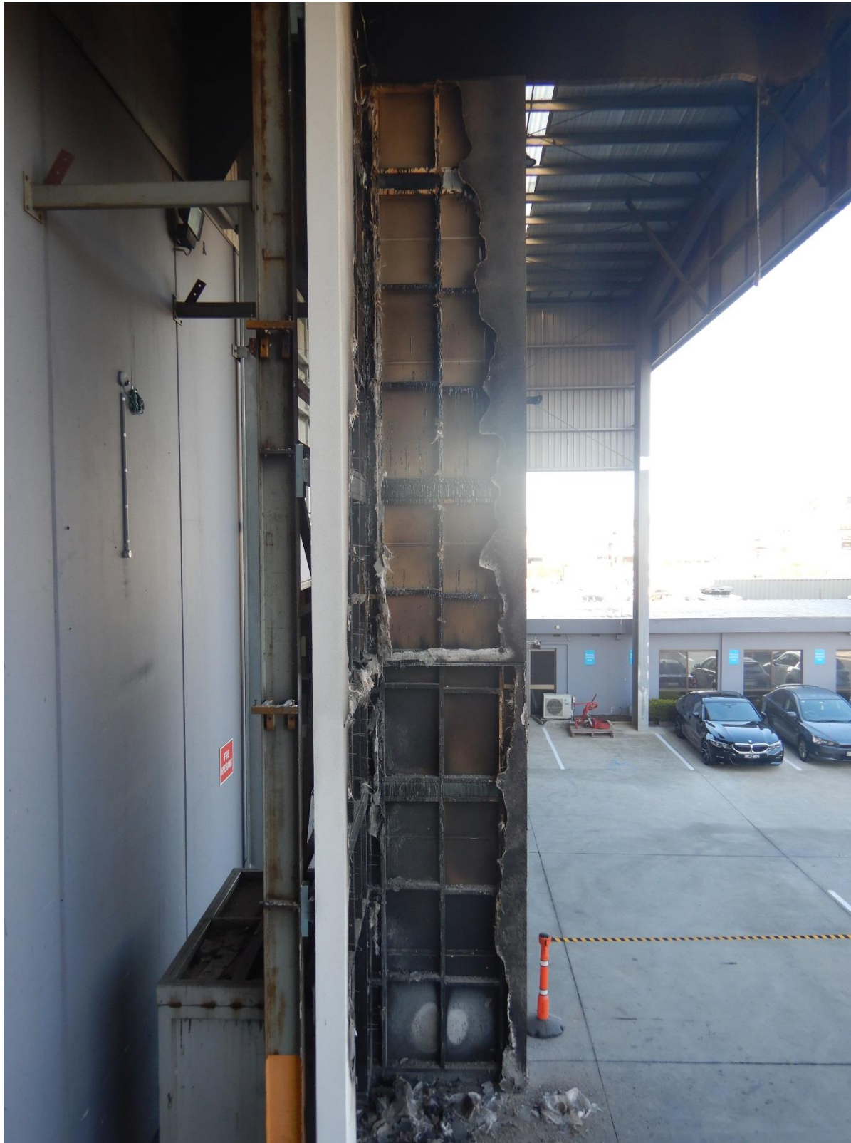
Figure 46 The post-test external wall system with severely heat damaged render removed – wing wall
