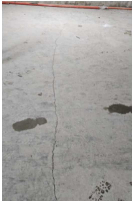
Figure 10: Crack forming in basement slab.
