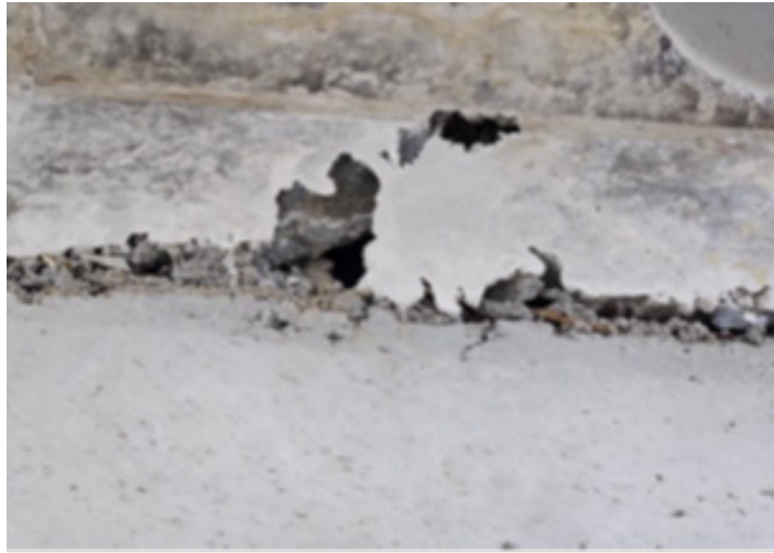
Figure 11: Honeycombing and exposed reinforcement bars.
