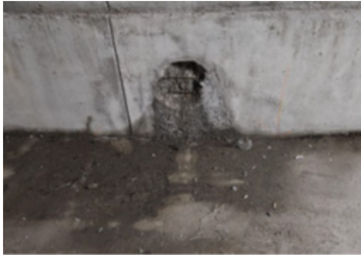
Figure 8: Exposed reinforcement bars and water leakage.
