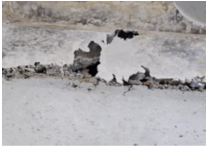
Figure 5: Honeycombing and air voids in shotcrete wall.
