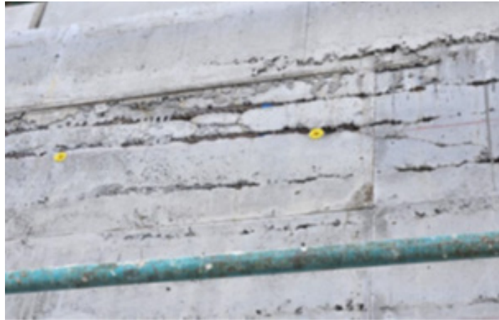
Figure 15: In situ wall with exposed reinforcement and honeycombing.
