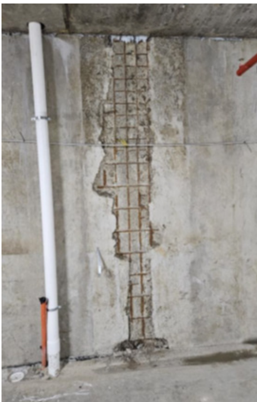
Figure 6: Damaged surface exposing reinforcement.
