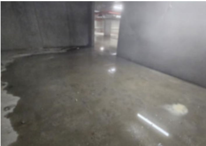
Figure 9: Excessive water ponding.
