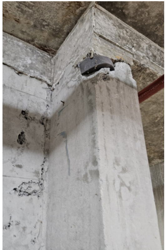
Figure 13: Damaged surface at ramp.
