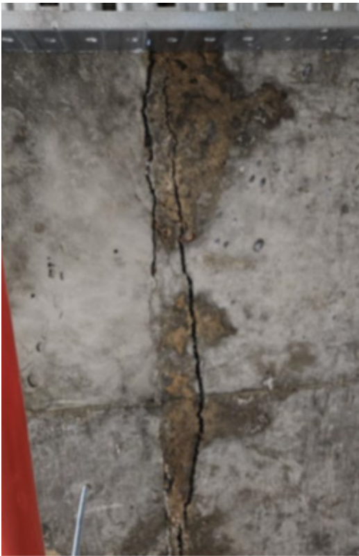
Figure 12: Cracks forming in soffit.
