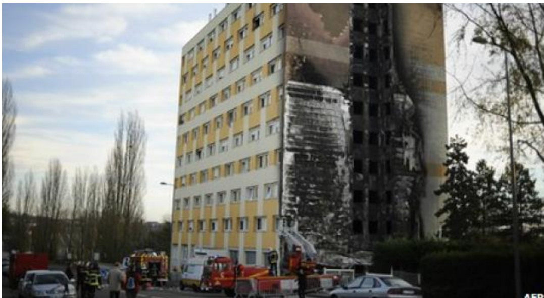
Figure 45 – Dijon France Immigrant hostel post fire damage [80]
